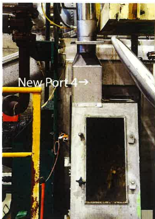
24-101: New Vacuum Port 4 Location
