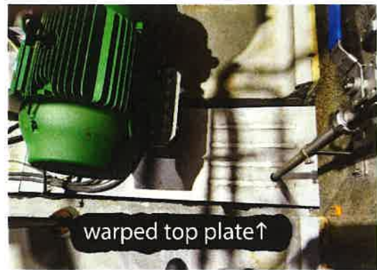
24-122: Conveyor between 12w and 12a
