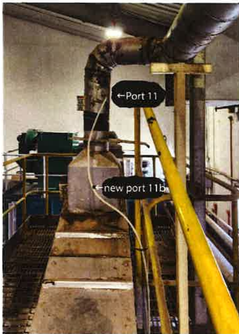
24-111: Driers Feed Conveyor Port 11
