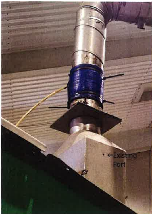
24-106: West side of Duct 13
