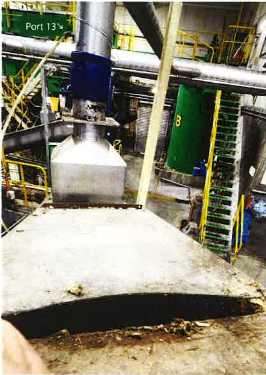
24-105: Existing port 13 location
