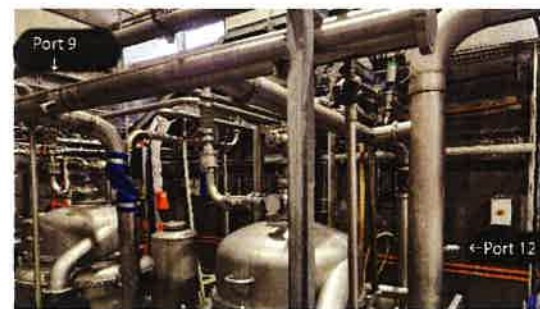
24-109: Port 9 to Duct 12 piping
