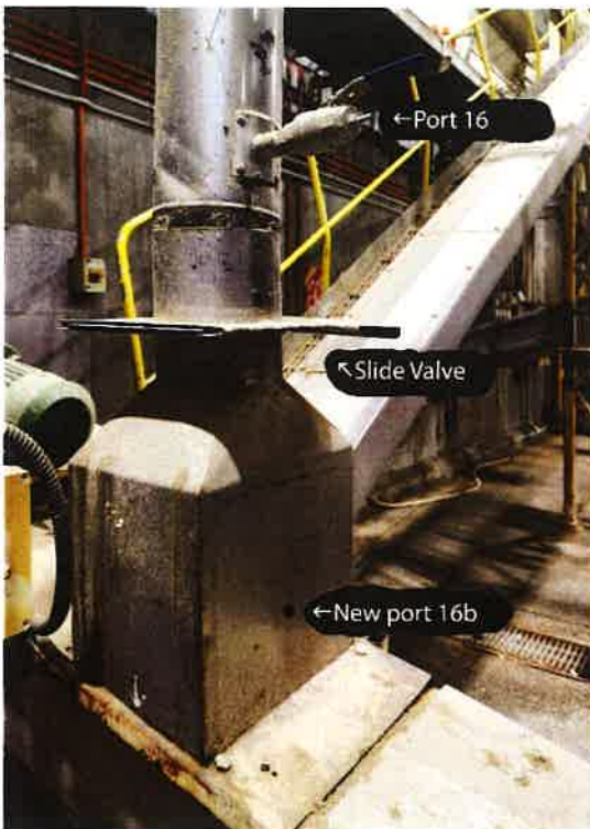
24-115: Meal Discharge Conveyor Port 16
