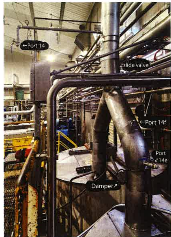
24-113: Decanter Feed Tank 2.11 ports
