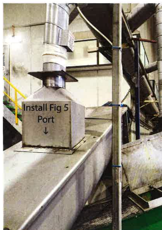
24-103: Drainer conveyor new Fig 5 flow measuring port location
