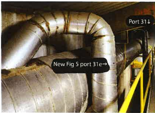
24-119: Ground meal bin ducting
