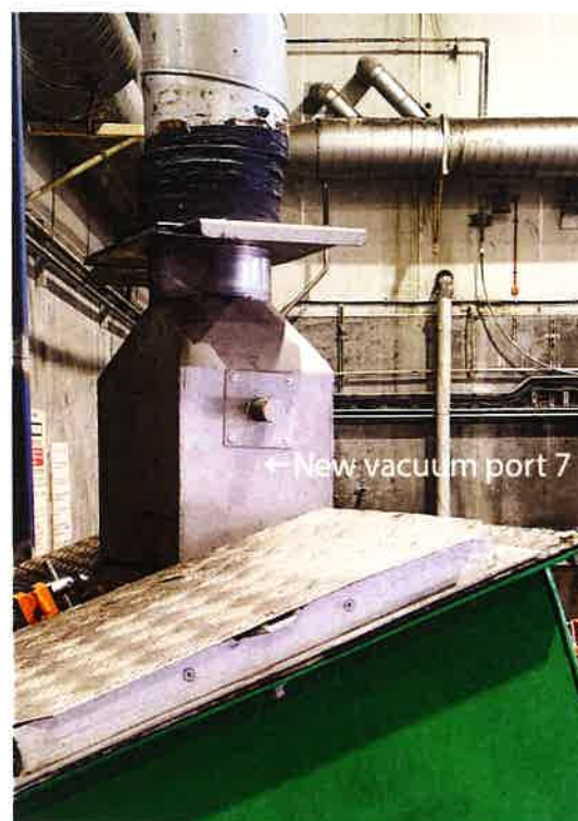
24-104: New vacuum port 7 location
